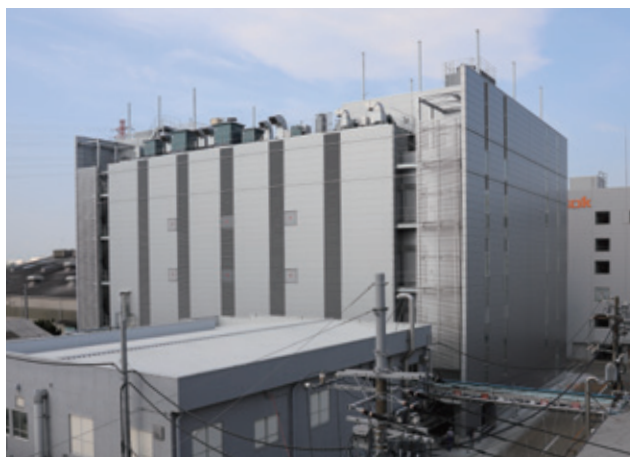
New C-1 Building (under construction) at the Sagami Operation Center will have a super clean room
